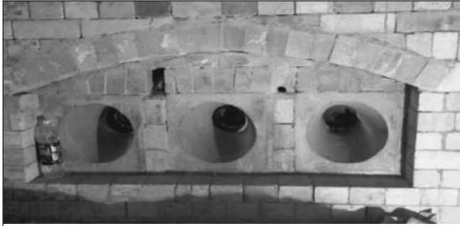
Refractory lining and burner blocks without coating
