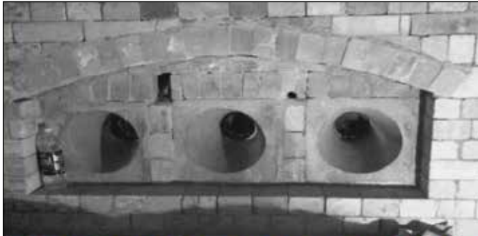
Refractory lining and burner blocks without coating
