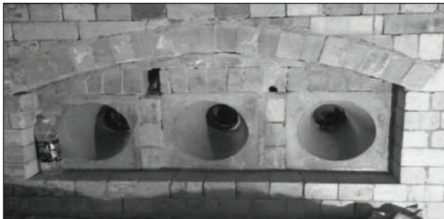
Refractory lining and burner blocks without coating
