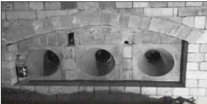
Refractory lining and burner blocks without coating
